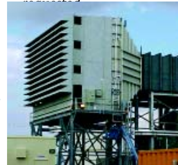
RIGHT: Evaporative cooler section is typically located behind filter section.
