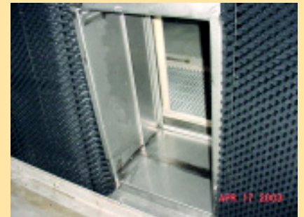
From the backside. The drift eliminator panels snug up to the sides of the door.
