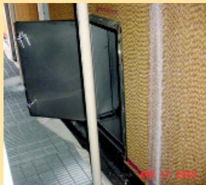
The 30"-high 'hobbit' door opens easily for access to the transition area behind the evaporative cooler media.
